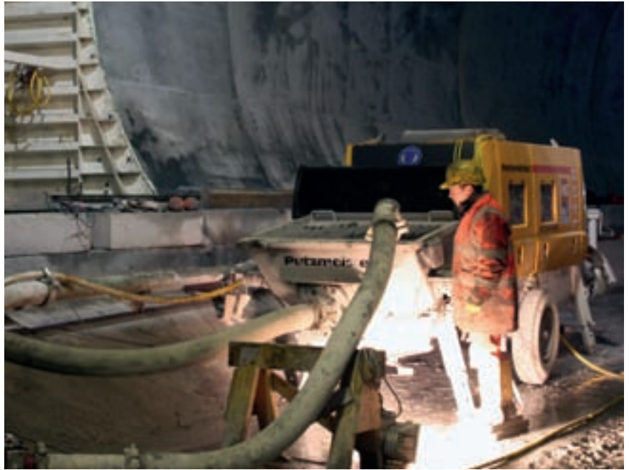
A hose was branched off from the delivery line and fed the BSA 1408 E at the arch formwork carriage
