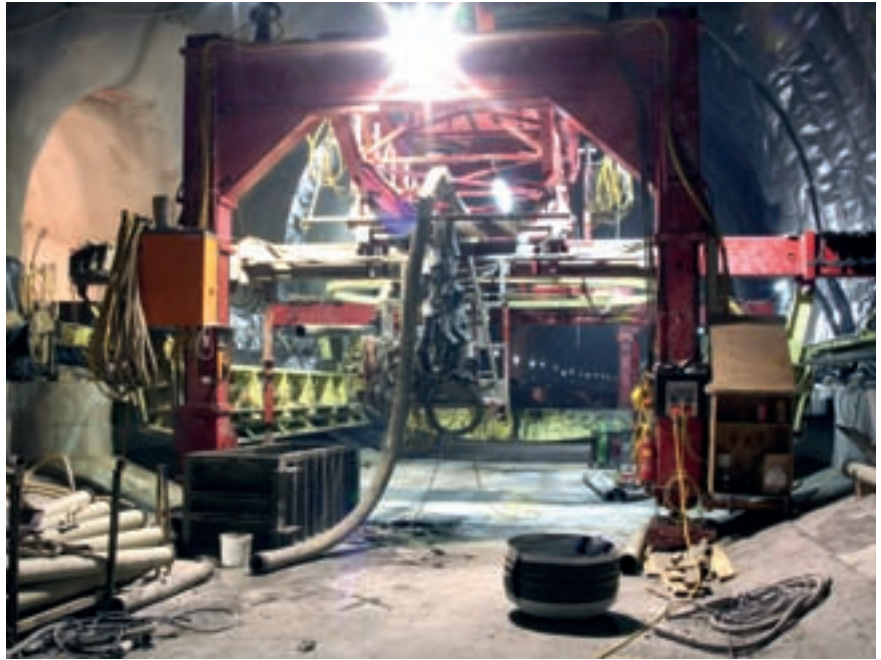
The formwork carriage at the front is the base formwork carriage. The prepared steel reinforcement can be seen at the end of this carriage.
