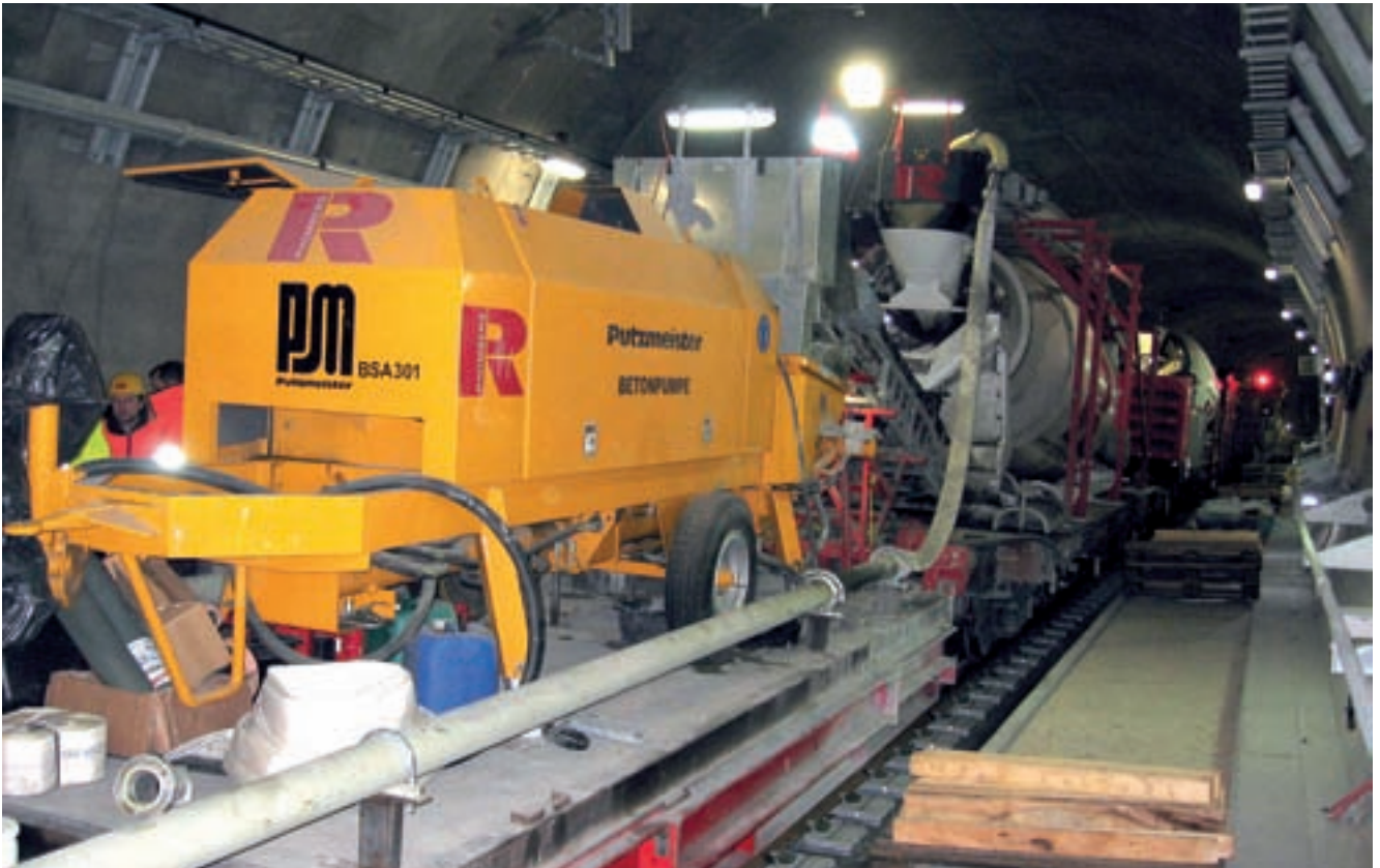
The concreting train with electrically operated concrete pump, which is fed via a conveyor belt
