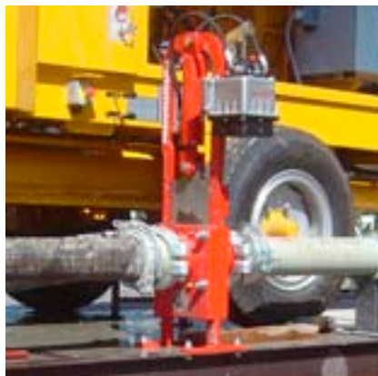
Between the concrete delivery and the cleaning process, a hydraulic manual gate valve has been installed to block the delivery line.
