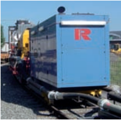
The main power supply is provided by a diesel unit with output of approx. 400 kW that is equipped with a soot particle filter for operating in the tunnel.
