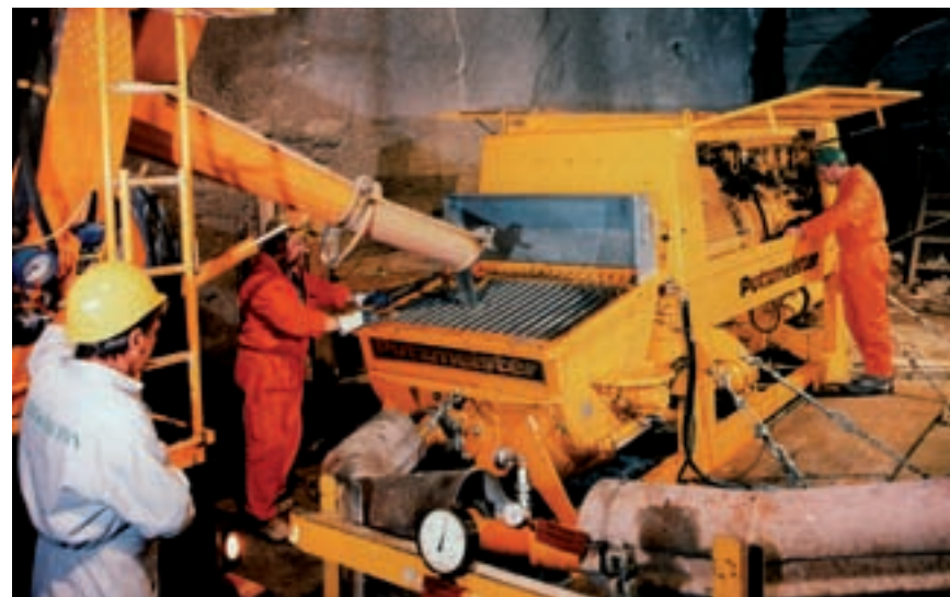
Protected delivery line and direct concrete pressure gauge. Pump anchored to the ground for long-term operation
