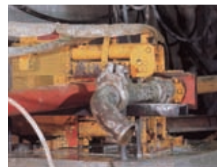
3-way gate valve for air-water cleaning using the sponge ball
