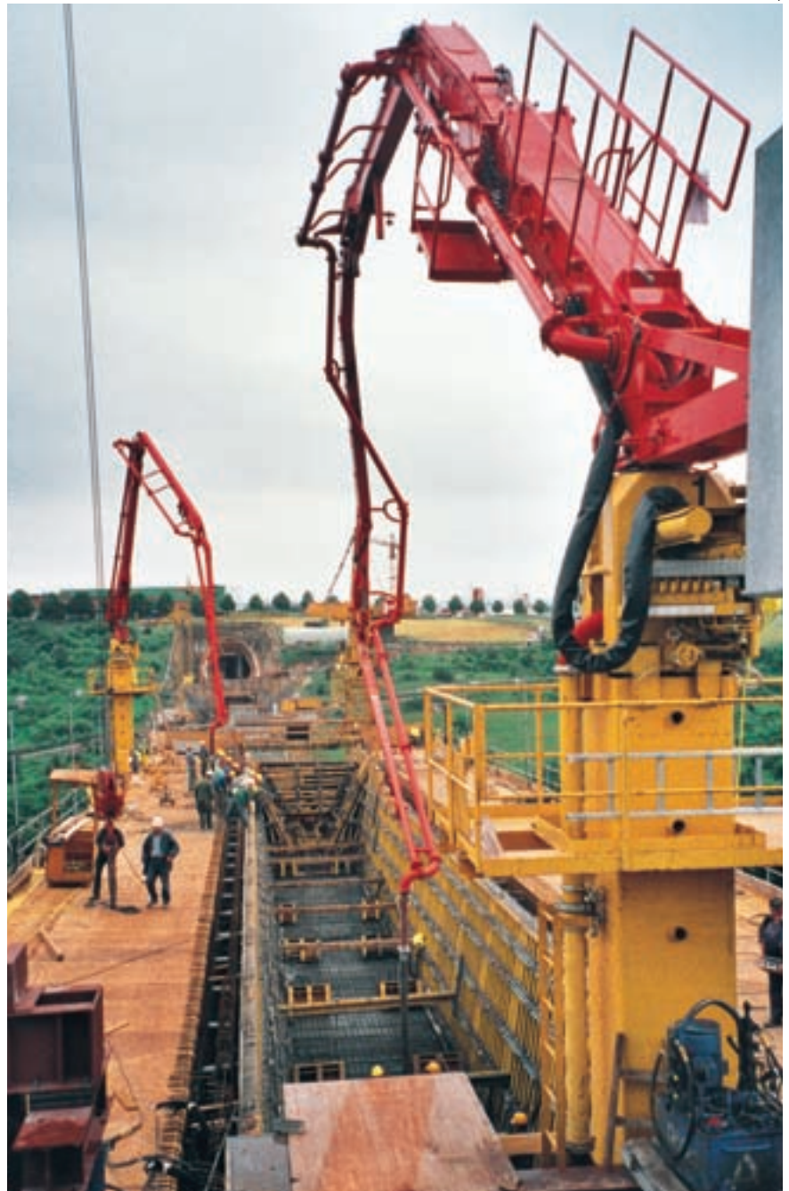
The two stationary booms MXR 32 (at the front) and MXR 24 concreting the bridge trough
