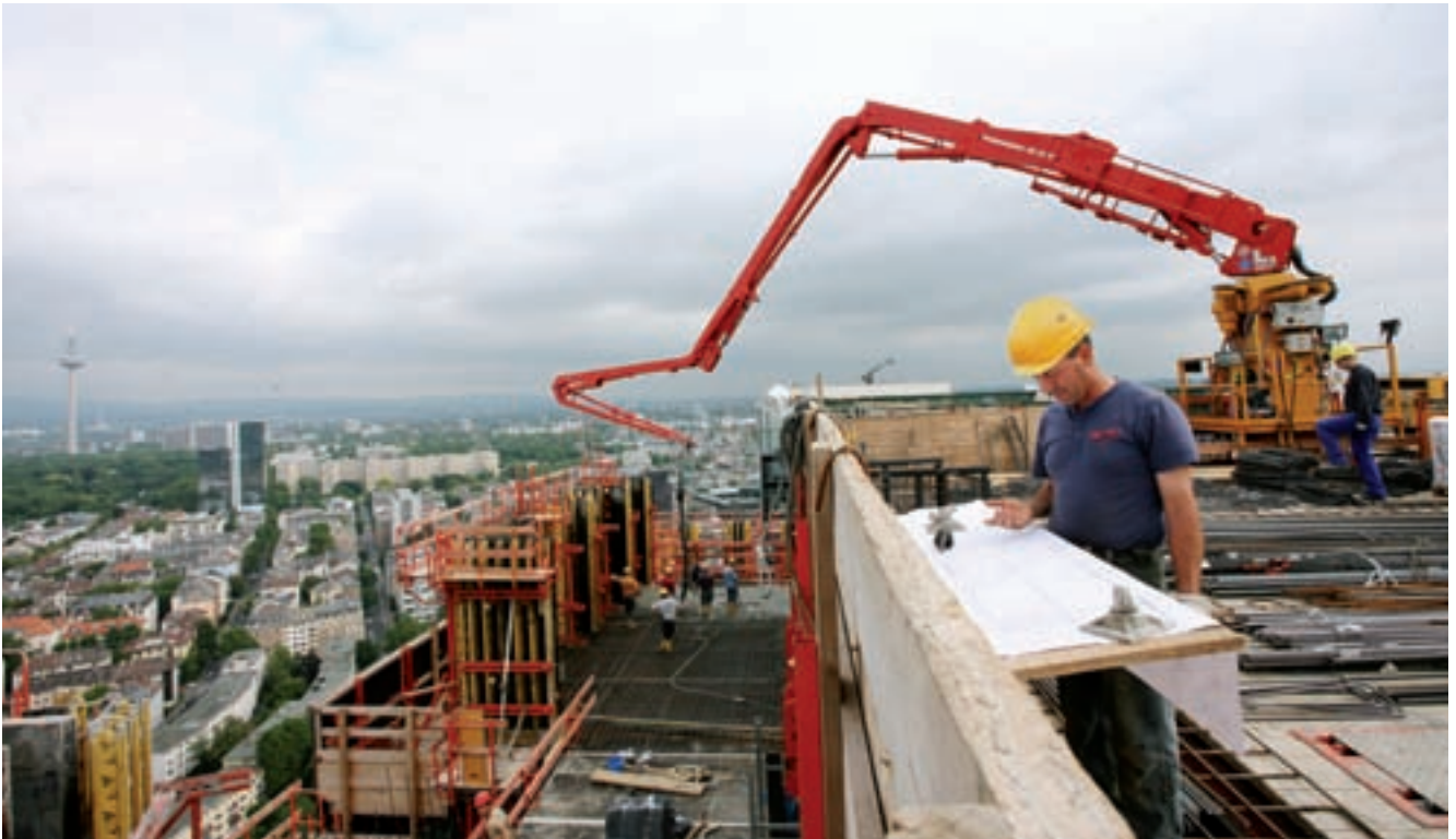
From a higher position, the PM stationary boom also distributes the concrete to hard-to-reach parts of the ceiling formwork
