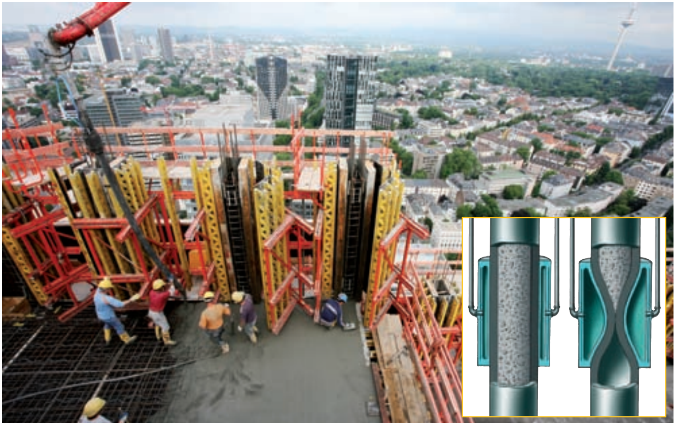
When the floors were concreted, approximately 100 – 120 m 3 concrete was placed within three hours, high above Frankfurt
