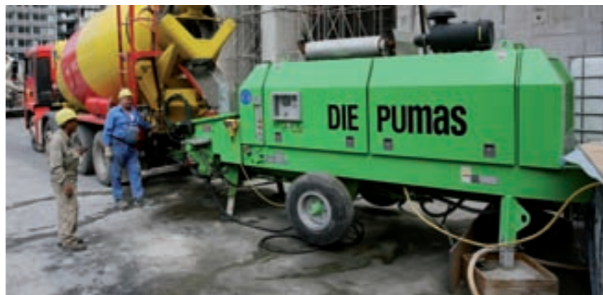
The BSA 2109 H D is connected to the 170 m high riser by means of an 80 m long horizontal delivery line
