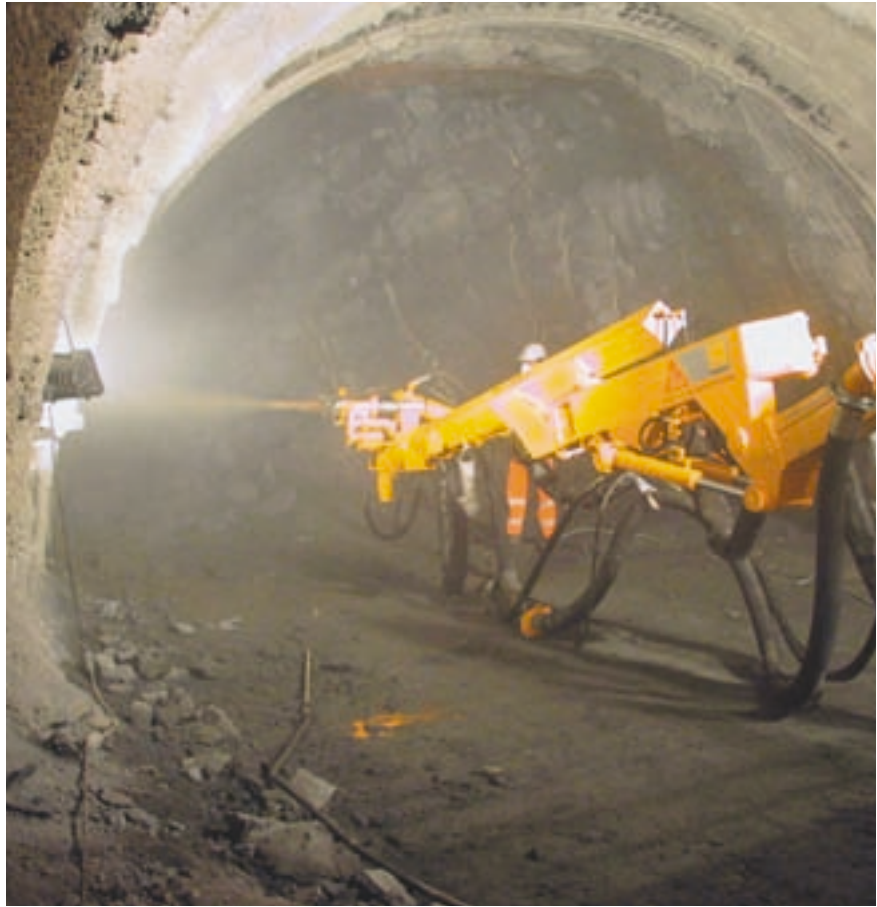
A WETKRET WKM 103 was used for wet shotcreting of the approx. 10 – 15 cm thick exterior shell.
