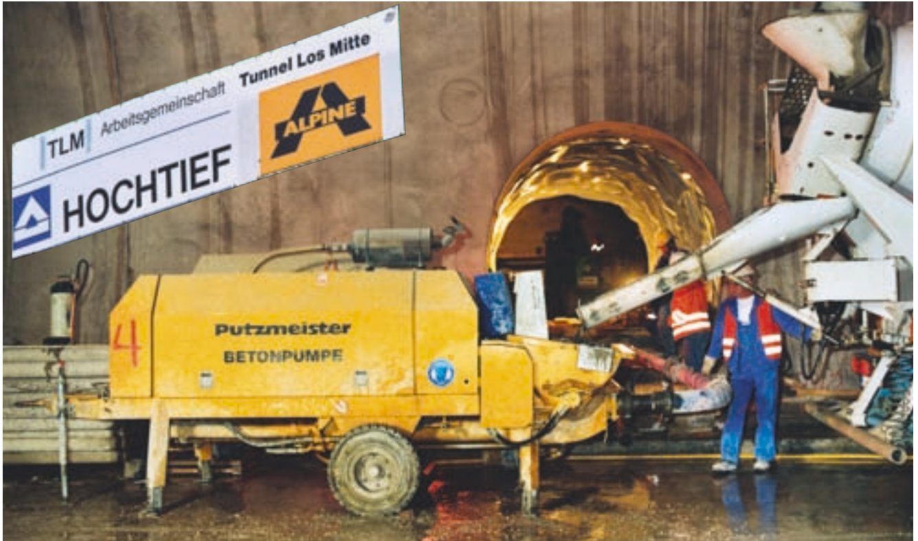
One of the 11 BSA's placing concrete in a cross tunnel in the Irlahüll Tunnel
