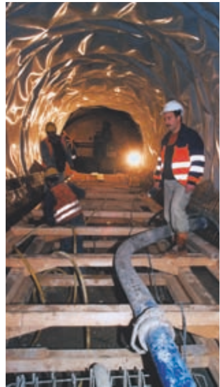
Some of the BSA concrete pumps are 400 meters away from the placement site
