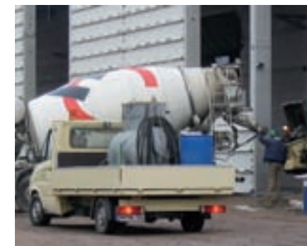
A mobile fuel station took over the task of providing the concrete pumps with diesel
