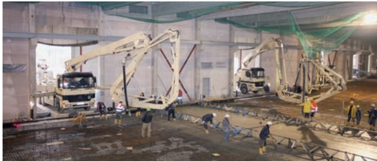
Up to five M 31-5s concrete the new DESY experimental building's base plate, which is 1 m thick, 24 m wide and almost 280 m long
