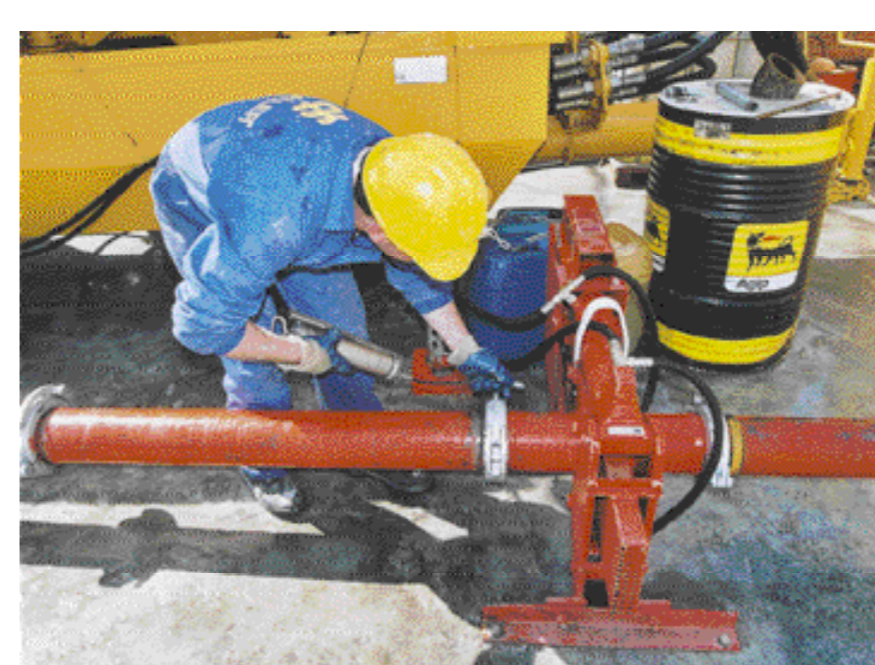
The gate-valve is also regularly lubricated
