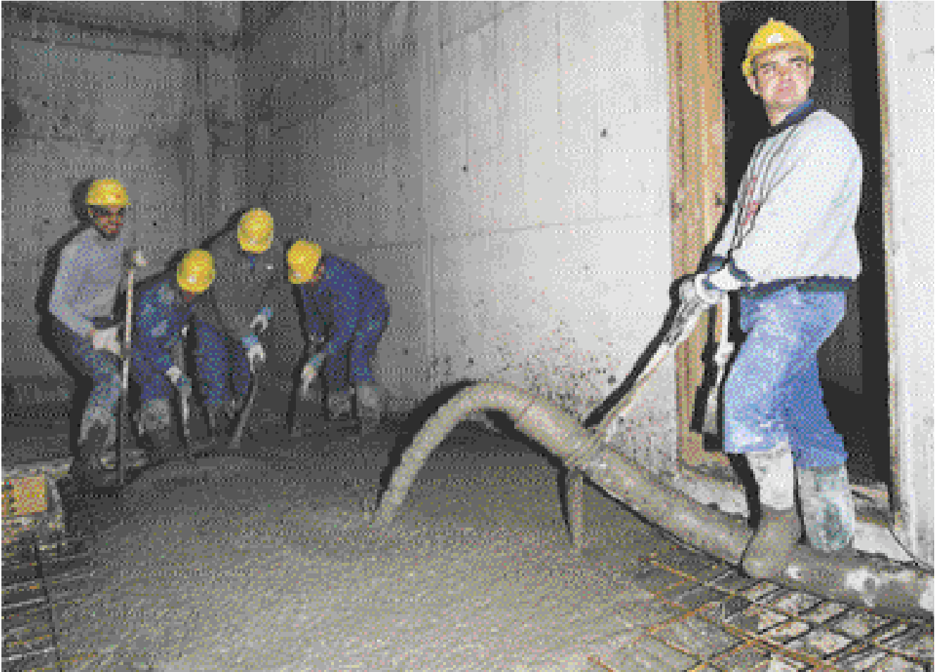
To place concrete on small surfaces, the pipeline to the boom is interrupted and flexible conveying hoses connected
