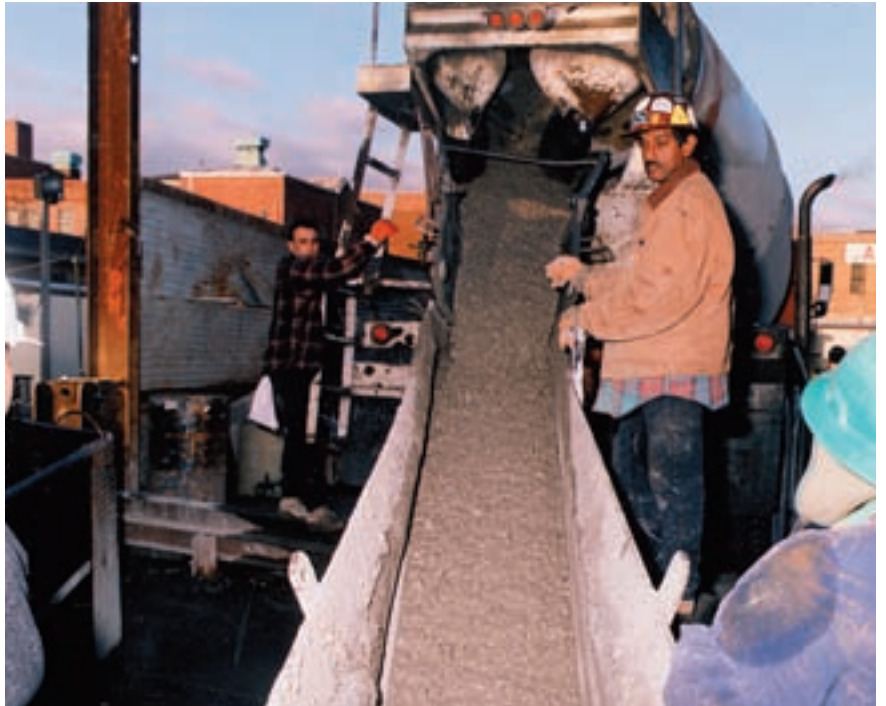
The concrete is “dropped” through a downward line into the gallery that is 165 m lower down
