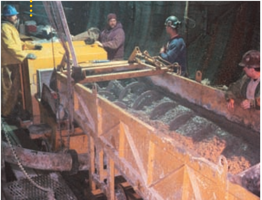
The Jumbo trough serves as an in-line mixer and "collecting vessel" for the concrete that is delivered in batches
