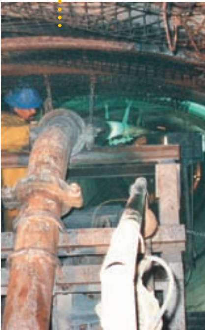
The delivery line is guided on roller bearings in the roof
