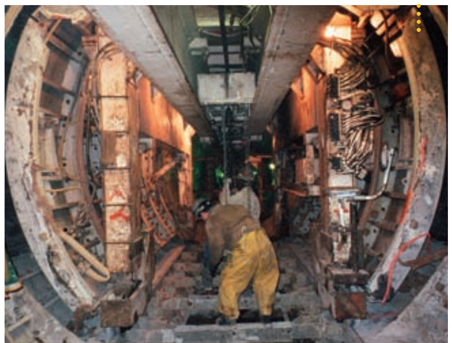
The formwork segments are continuously moved in the direction of the shaft start
