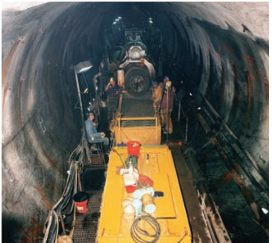
Transport wagons (in the rear) pass the concrete to the Jumbo trough for remixing before the BSA 2100 HD-E (in the foreground) takes over the pump conveying
