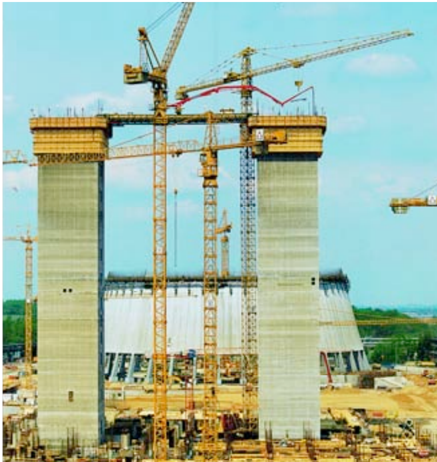
The concrete placing boom MXR 32 was in the center point of this remarkable construction concept
